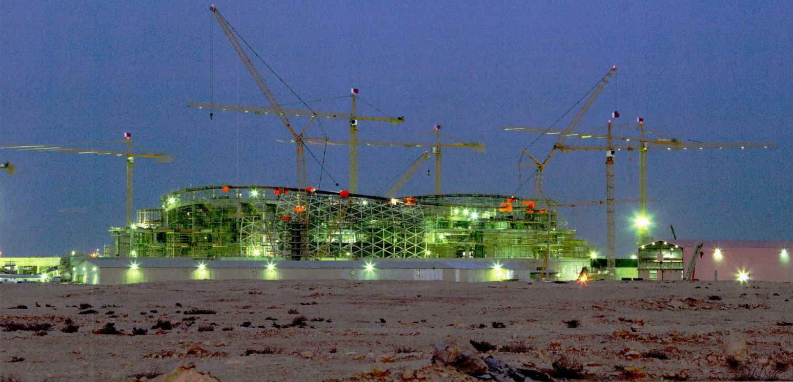
Construction of a new stadium near Lusail, Qatar. Credit: Philip Lange / Shutterstock.com
